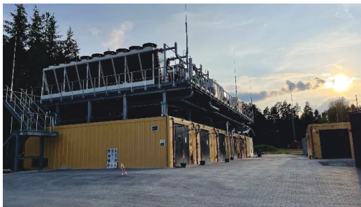
Fig 5: Picture of the modular BALIS test field covering a surface area of 2000 m 2 .
